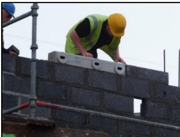
Figure 19: Installing Swift boxes as part of the fabric of the wall. Photo: Lynda Huxley (Swift Conservation Ireland).
